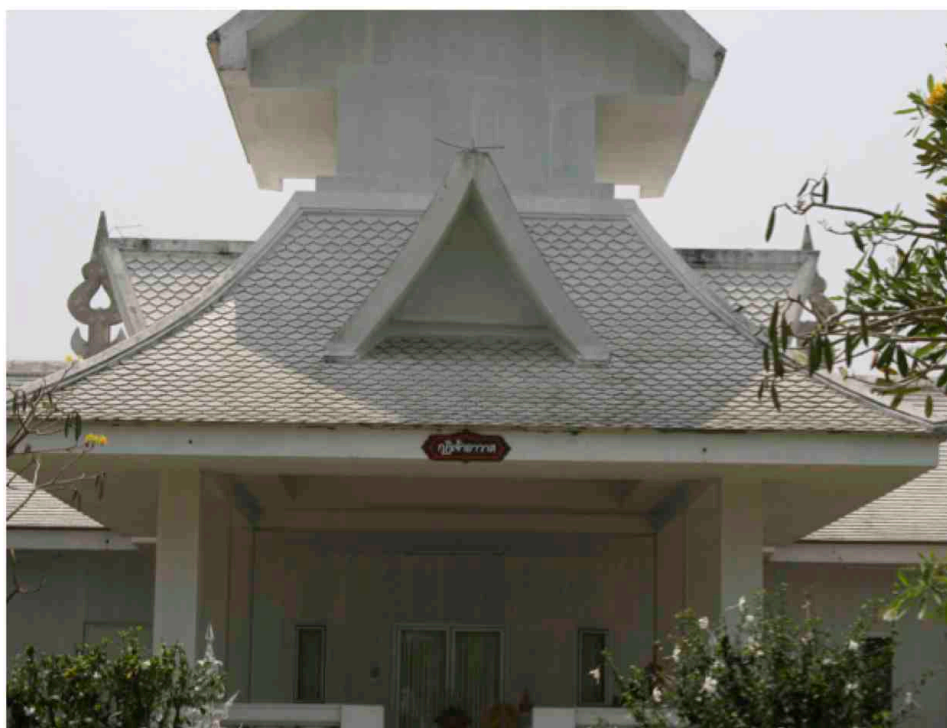
Fig. 34. Watermarks still visible even after cleaning the roof, March 2010.
