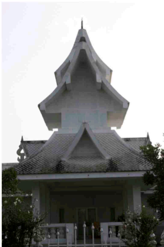
Fig. 33. Water stains and mold on kuti , December 2008
