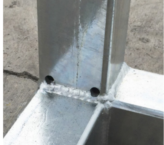
(b) Holes near weld at corner regions of a RHS connection
