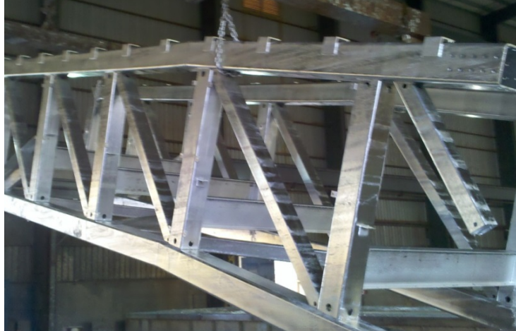
(a) Galvanized tubular truss with holes
