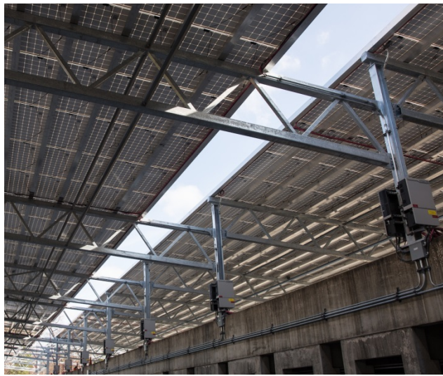
(a) Roof truss at T Rowe Price Parking Garage Baltimore, MD, United States
