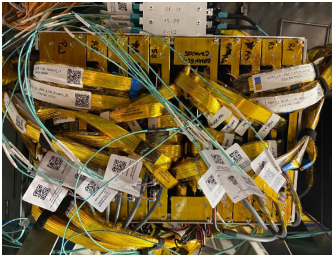
Figure C.3: Rim crate with everything connected and with proper cable management. On top the small fiber box can also be seen.
