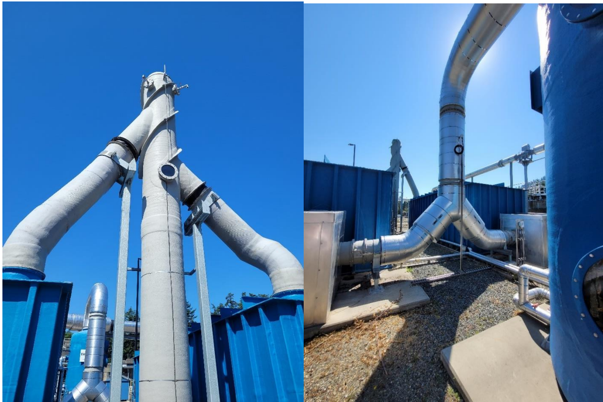
Figure 29: (Left) Photo of Bioreactor exhaust stacks, sample point 9. (Right) Photo of Bioreactors showing ductwork from raintower which is sample point 8.
