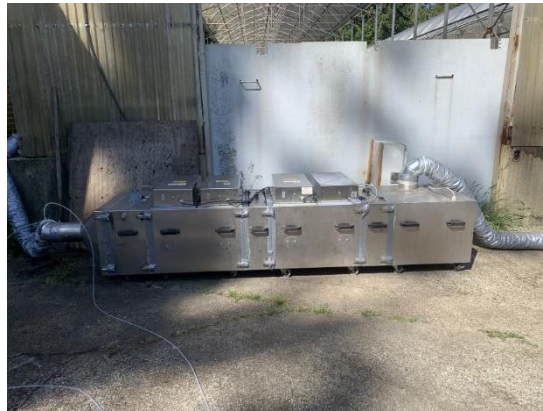
Figure 16: Photo of Advanced UV oxidation unit for odour control, Inlet on the left of unit and outlet at the right.
