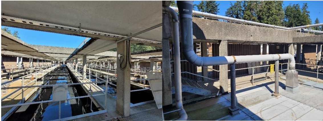
Figure 27 (Left) Photo of primary treatment sedimentation. (Right) Foul air collection from primary treatment, ductwork is sample point 4 and is plumbed to the Bioreactor odour treatment system.
