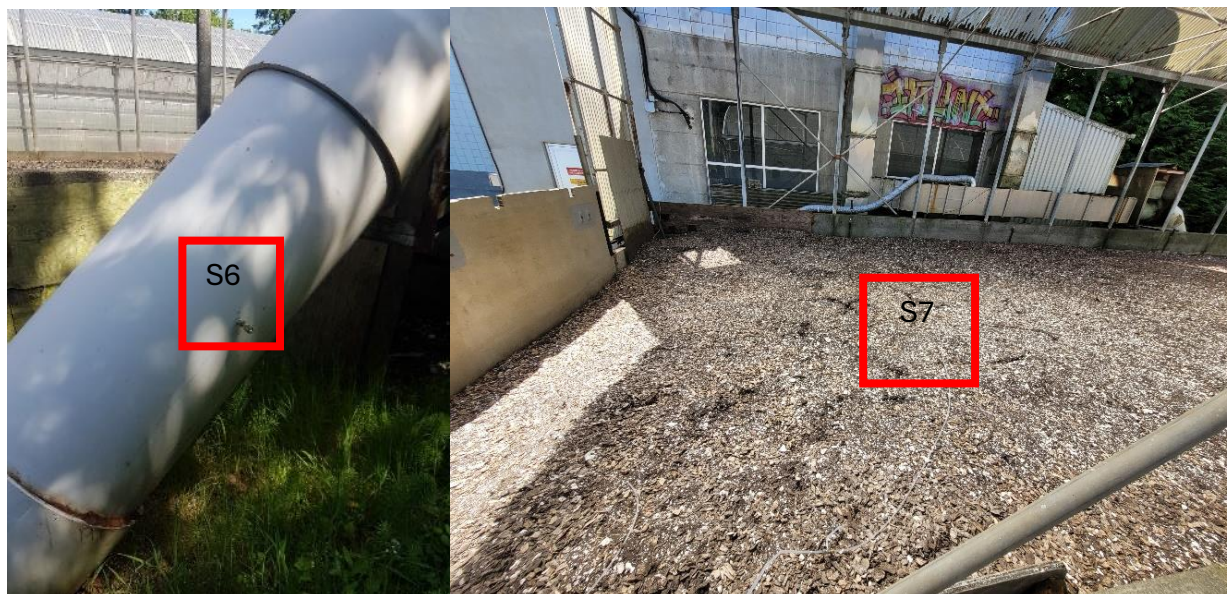
Figure 12: (Left) Photo of ductwork after de-wetting, sample point 6. (Right) Photo of Biofilter, sample location 7.
