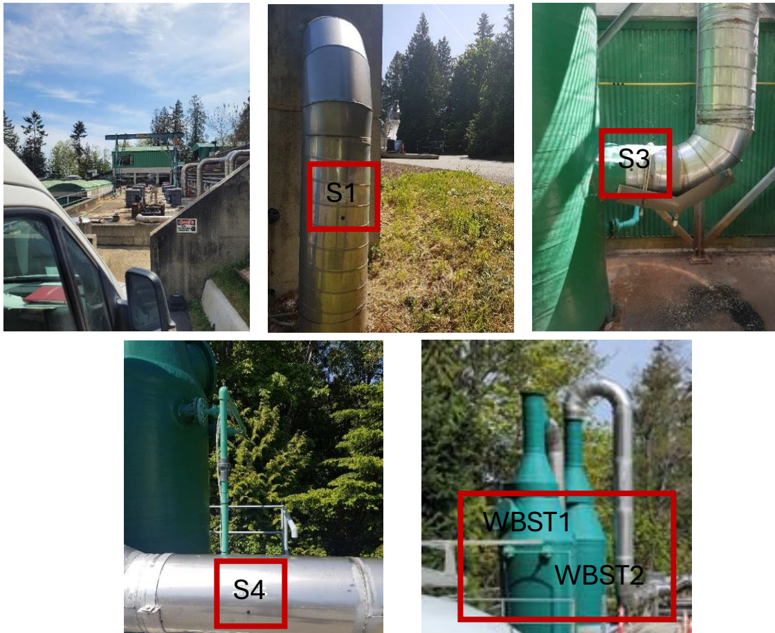
Figure 1: (Top-Left) Photo of ATADs treatment location at WWTP1, (Top-Right) Ductwork coming from ATADs foul air, sample point 1. (Bottom-Left) Photo of Sample point 3 ductwork coming from WBST1 into WBST2, (Bottom-Mid) Photo of ductwork sample point 4, leaving WBST2.
