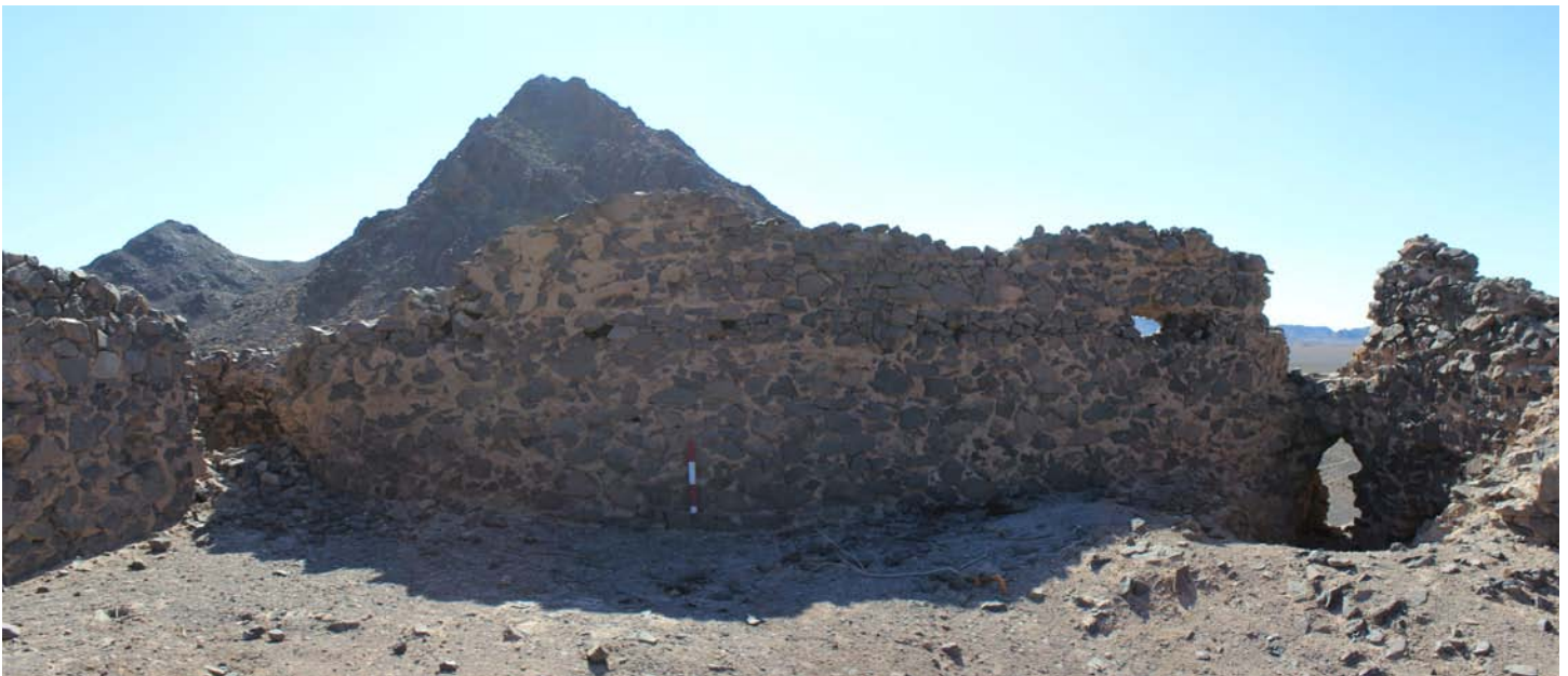
Figure 4-63: Inside Qal'ih Zari, view to the western wall. Note the small joist holes in the upper half of the wall. Credit: Author.
