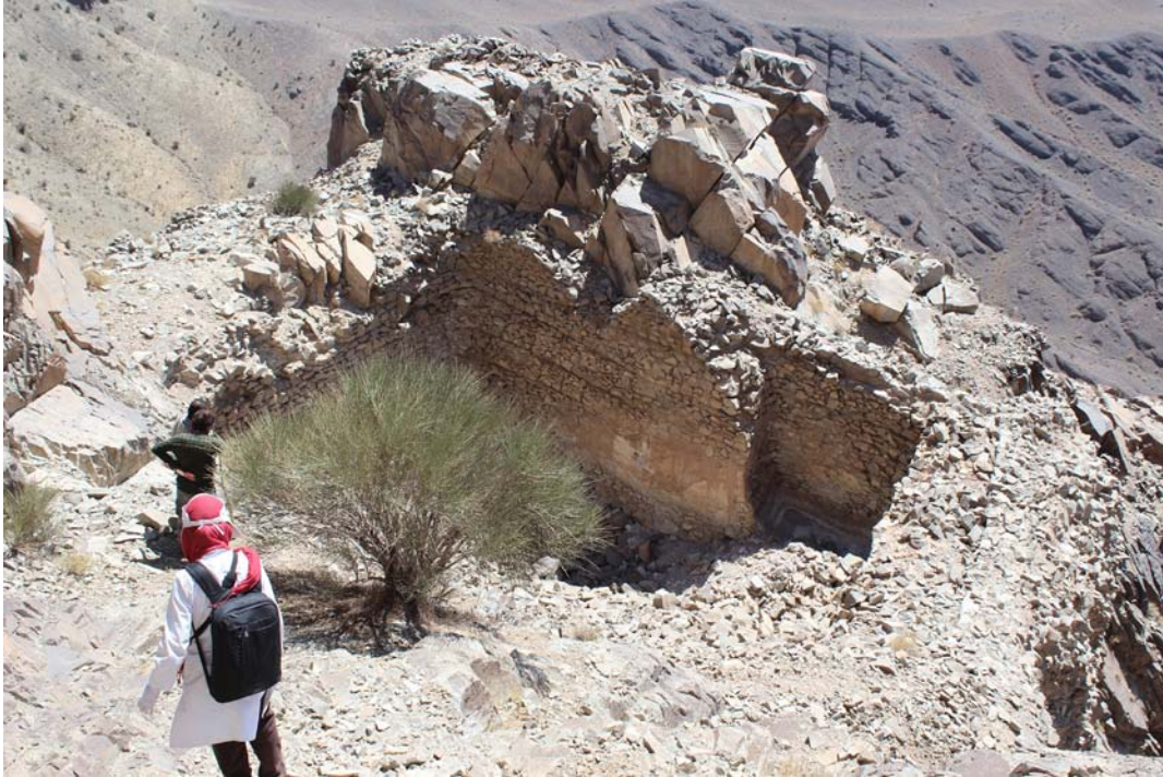
Figure 4-51: Qal'ih-Rustam of Khusf, the large cistern in section B, viewed from the northwest. Credit: Author.
