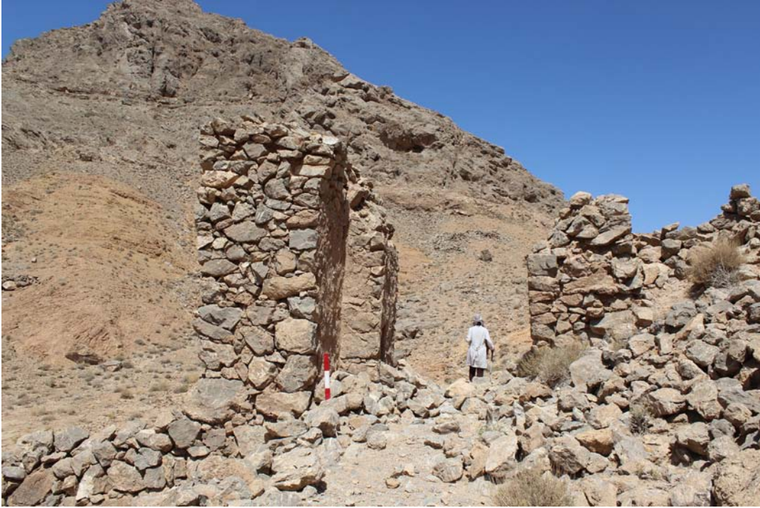
Figure 4-74: The main gateway of Qal'ih Kafaran viewed from the exterior. Credit: Author.
