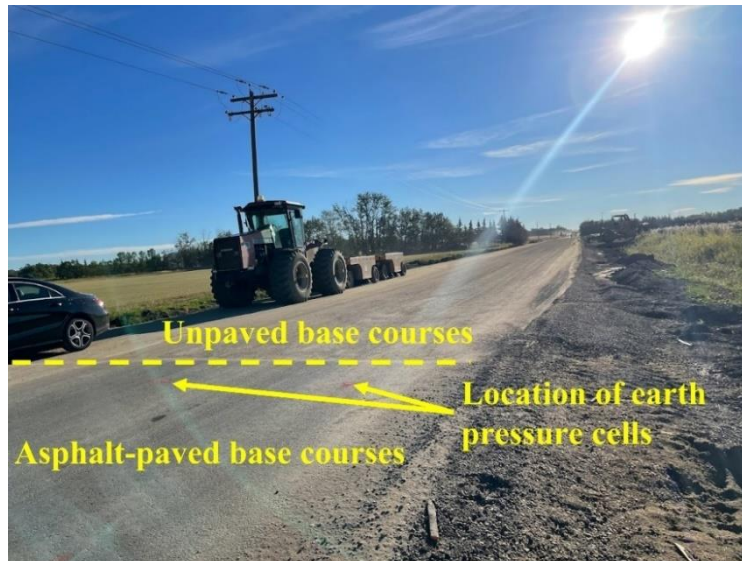
Fig. 5.33. Photograph of the location of earth pressure cells in geocomposite section
