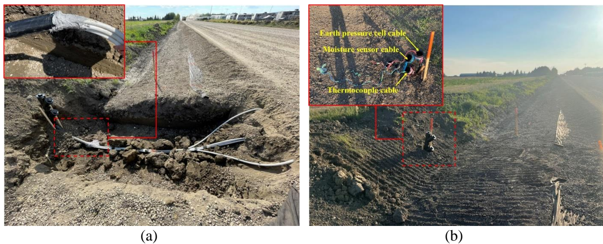
Fig. 5.21. The cable access terminal for the 4-inch geocell section: (a) trench excavation and (b) terminal tower installation
