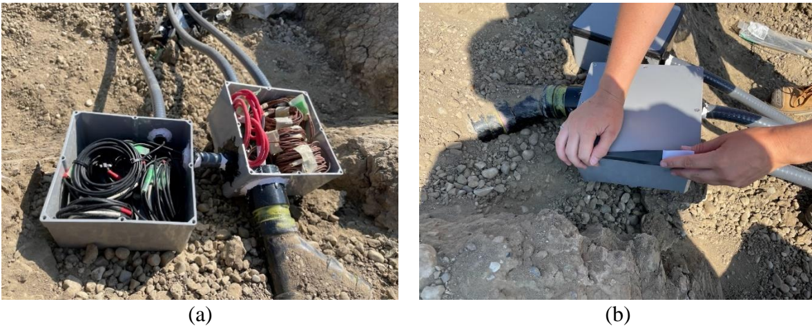
Fig. 5.23. Access boxes: (a) extra cables and (b) box closure
