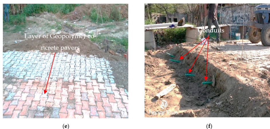
Figure 5. Step-by-step deployment of wastewater treatment system at Mehat car wash site: (a) creating a 5 m × 0.8 m trench; (b) installing Silva Cells® in the trench; (c) planting poplar trees in the post of Silva Cells®; (d) filling the entire trench with coarse aggregates ranging 10–20 mm; (e) laying geopolymer concrete pavers over the layer of Silva Cells®; (f) installation of conduits for the outlet of treated wastewater.
