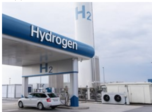
(c) Hydrogen refueling station (HRS)
