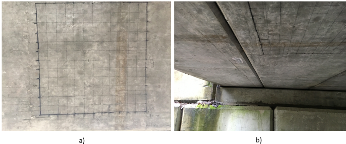
Figure 34: GPR and Profoscope tests on the bottom of the bridge deck slab; a) Test grid, b) Test Site SI-3006A
