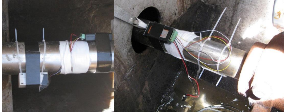
Figure 26: Strain gauge installations
