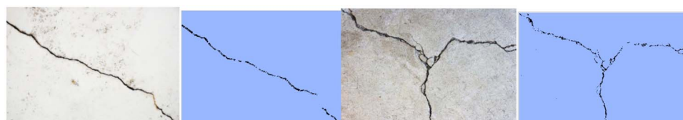
Fig. 3. HSV thresholding crack output
