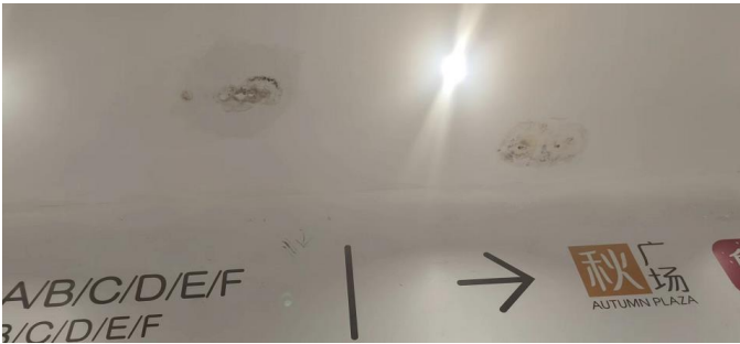
(C) MOLDS AND WATER LEAKAGE INSIDE A SHOPPING MALL
