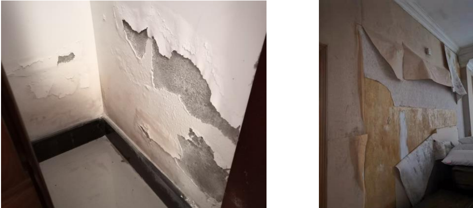
FIGURE 1 (A) MOLDS GROWTH AND WALL PAINT DETERIORATION (B) WALL COVERING PEELS OFF
