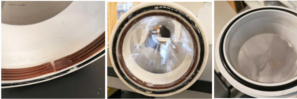
FIGURE 42 (A) WEATHER STRIP INSIDE COLUMN (B) WATER RESISTIVE GLUE (C) O-RING ONLY
