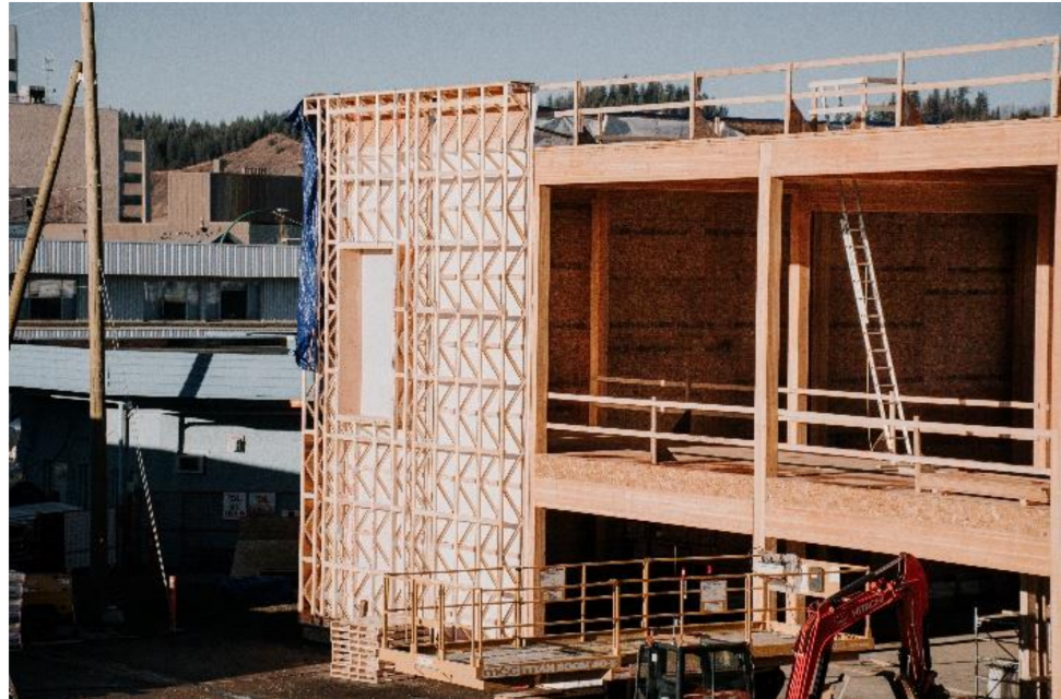
Figure 1. Wood Innovation Research Lab glulam post and beam structural system with vertical truss wall panel to be insulated on site.
