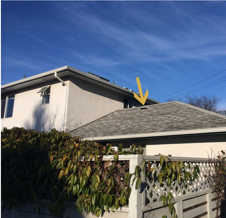
Figure 8 – Lower sensor location indicated by yellow arrow. Sensor sat on top of roof vent.
