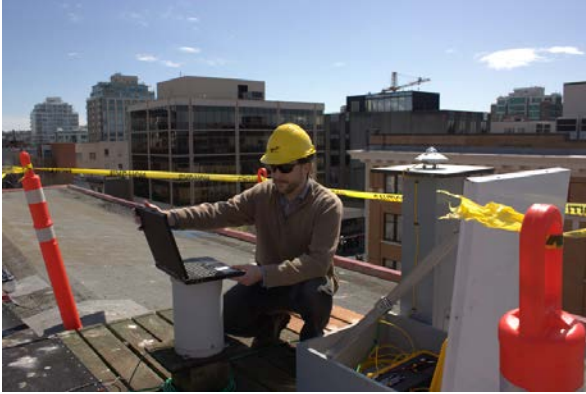
Figure 9 - Pedestal, pyranometer, and datalogger being programmed on city hall's rooftop.
