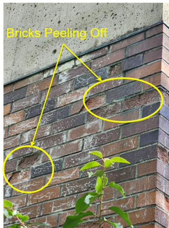
Figure 2. Bricks Peeling off MacLaurin Building in University of Victoria, BC, Canada
