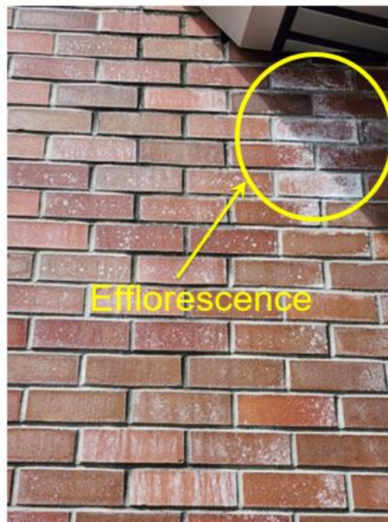
Figure 4. White Crystalline Coating on Brick Wall of Medical Science Building in UVic
