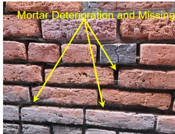
Figure 1. Mortar Deterioration in Fan Tan Alley, Victoria, BC, Canada
