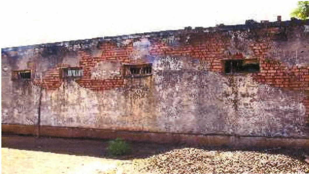
Figure 4. The rear view of the main structure of Namikango CBCC Centre showing the dilapidation as well as the high positioning of the windows
