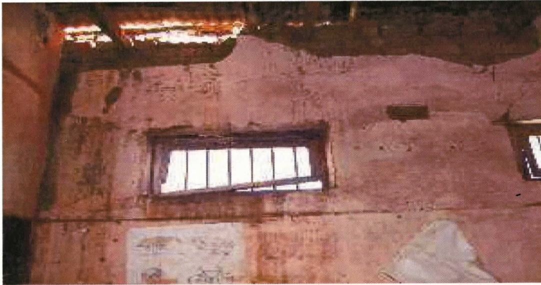
Figure 5. Part of the roof and window section of the room, which houses the children at Namikango CBCC Centre: Note the high, narrow windows and the large hole in the roof.
