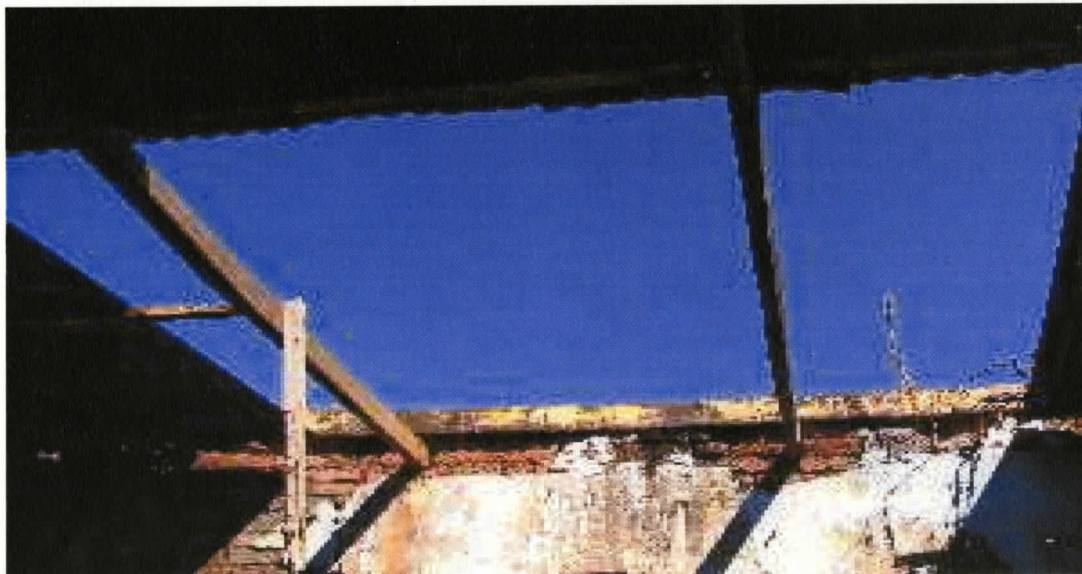
Figure 6. This figure shows part of the falling roof over a room adjacent to the room in which children gather for their activities at Namikango CBCC Centre.
