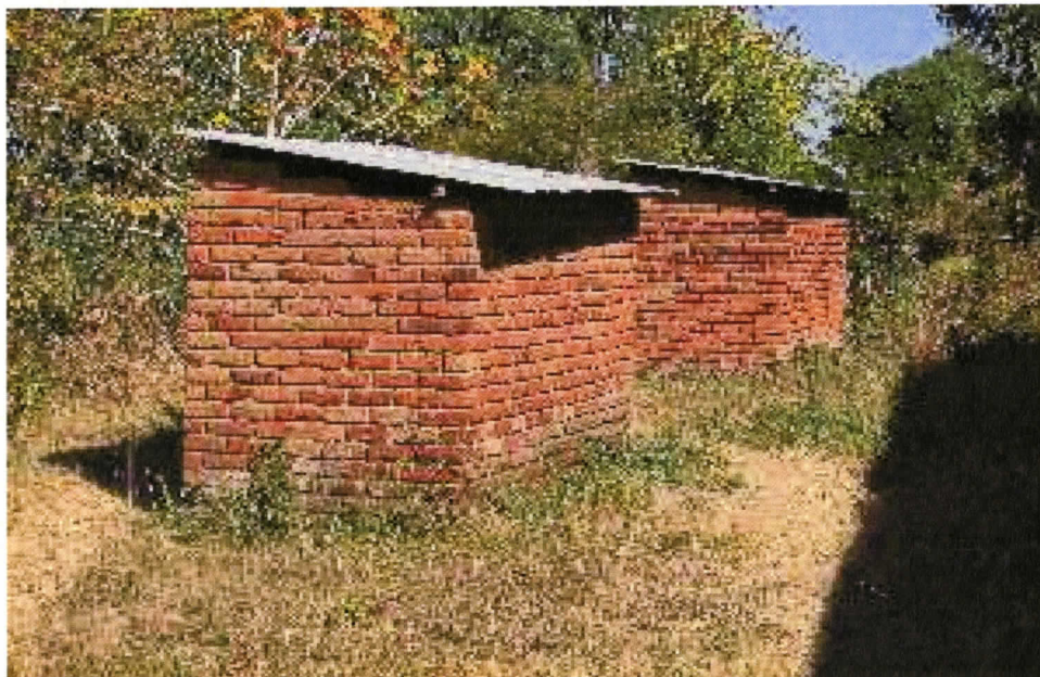
Figure 27. Two pit latrines each with two separate entries constructed about 30 metres away from the mains building at the Village-to-Village CBCC Centre.
