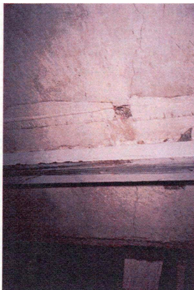
Longitudinal Crack at Underside of Deck Slab near Transverse Edge Stiffener
