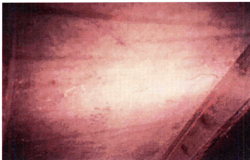
Figure 4.10 - Cracking Pattern on Bottom Surface of Panel 1
