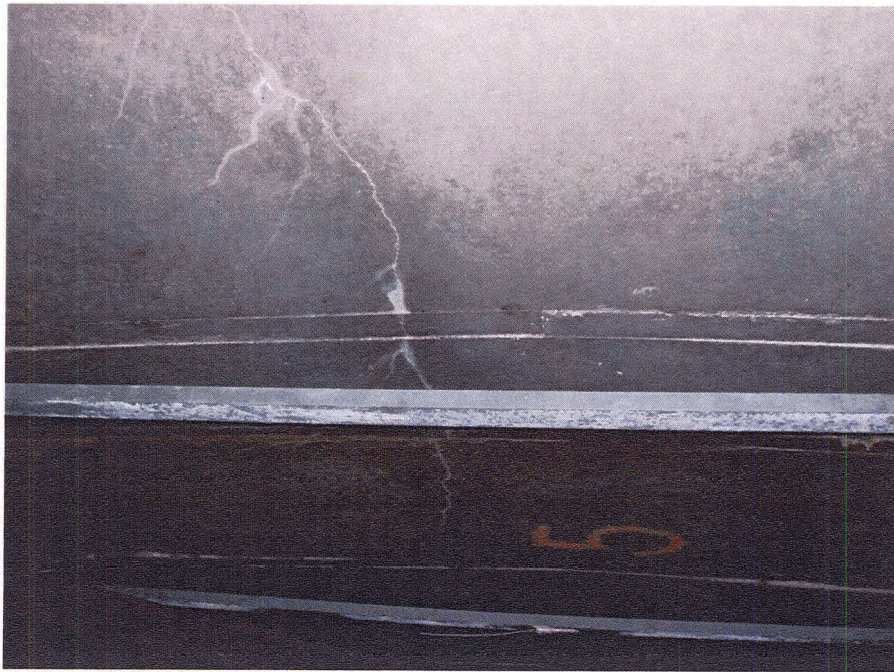
Figure 4.37 - Longitudinal Centre Crack on Bottom of Panel 5 Strain Gauge 5 can be seen on Steel Strap in Background
