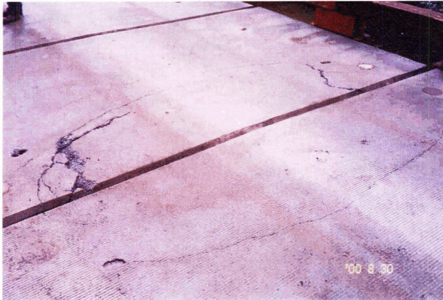
Figure 2.3 - Slab Failure at Unconfined Edge
