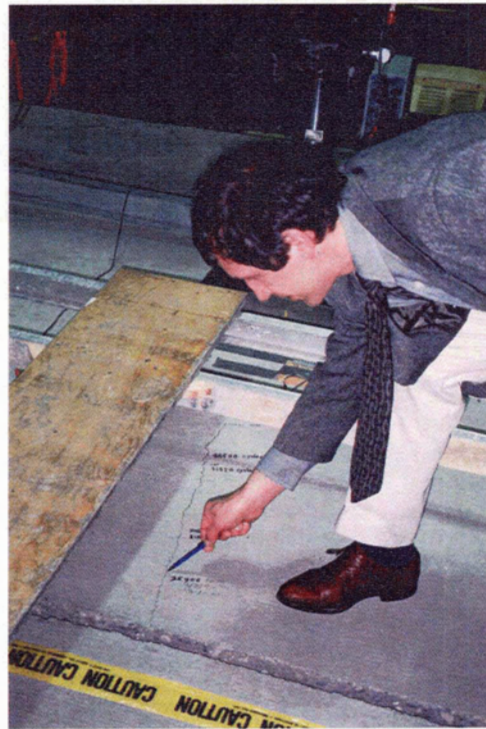
Figure 4.11 - Progression of Cracking on Top Surface of Panel 1
