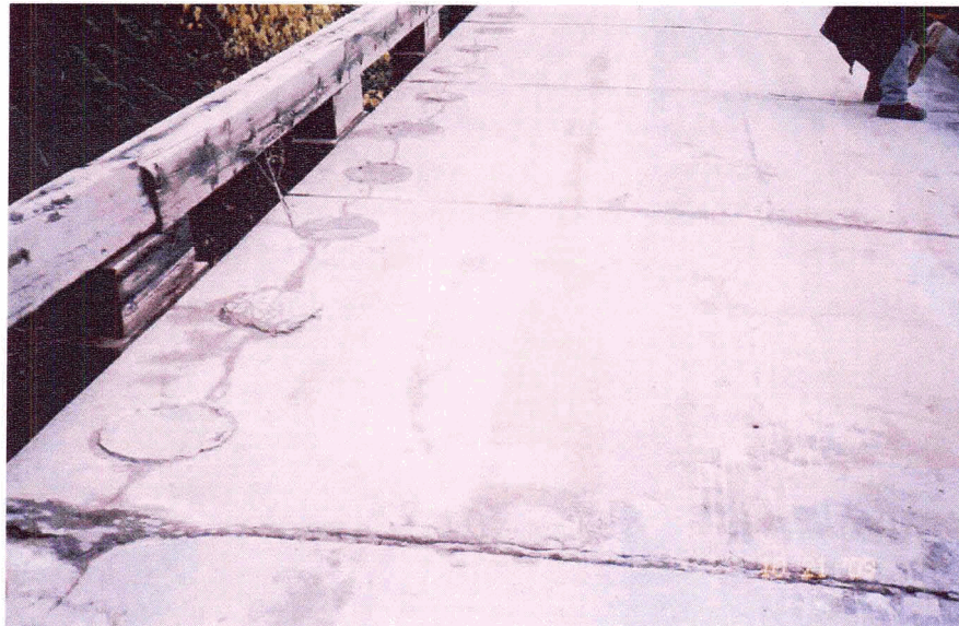
Figure 4.38 - Secondary Cracks at Grout Pockets
