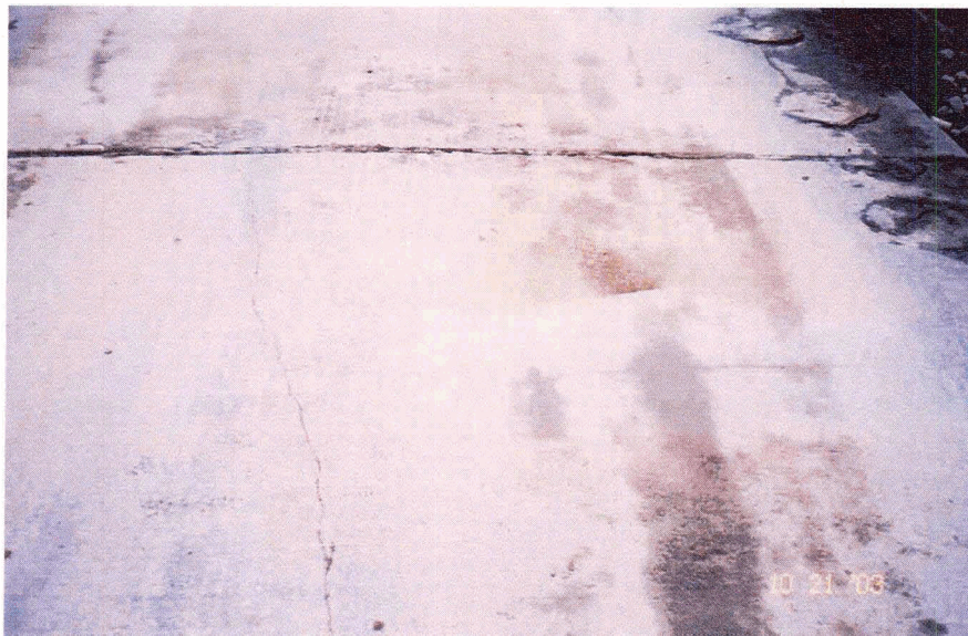
Figure 4.36 - Longitudinal Centre Crack on Top of Panel 8
