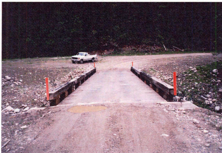
Deck Cleaned for Review of Crack Development
