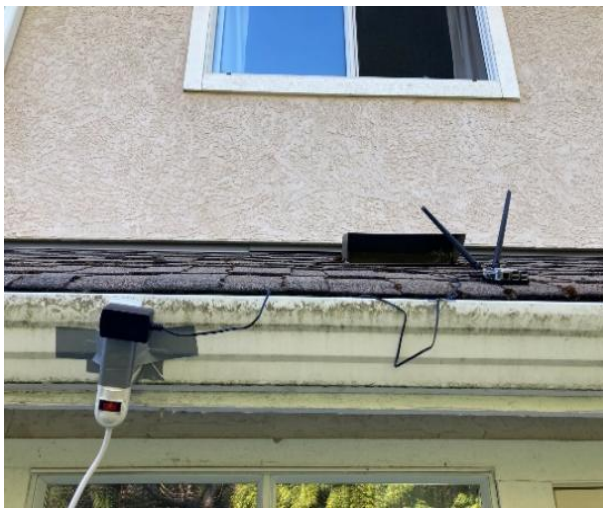
(c) Gateway deployed on the roof
