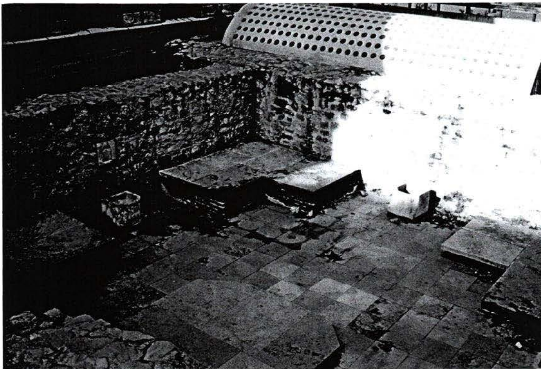
Figure 122: Hot room with the göbek taşı and sofas in the Bath of Memi Pasha.
