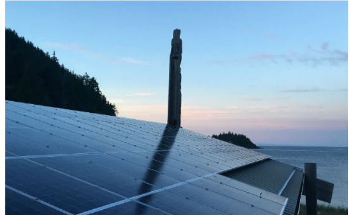
Solar installation on the roof of the Haida Heritage Centre in Haida Gwaii (Photo credit: Dana Cook, with permission).
