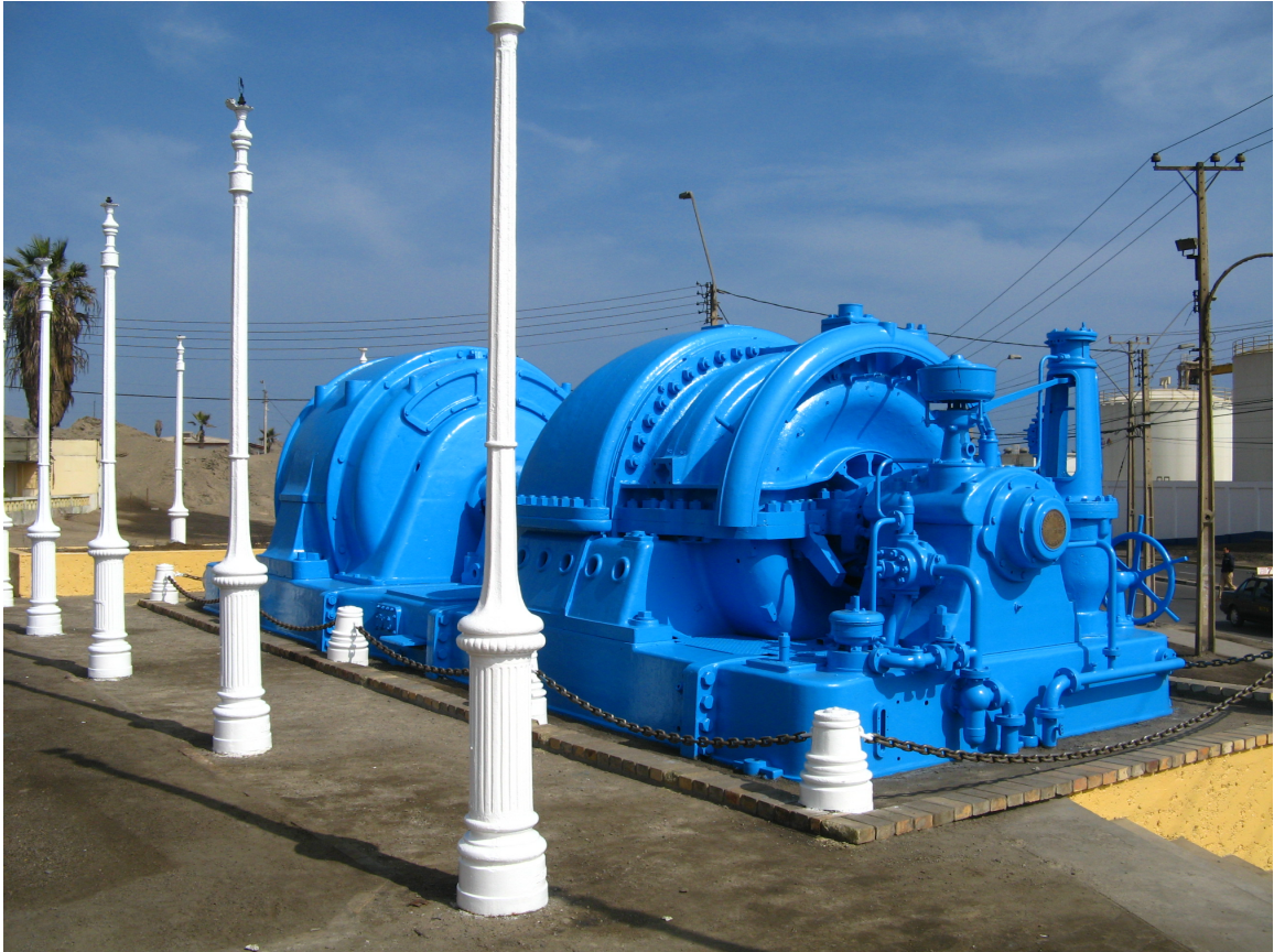
Figure 1.5: A steam turbine that has served for more than fifty years.
