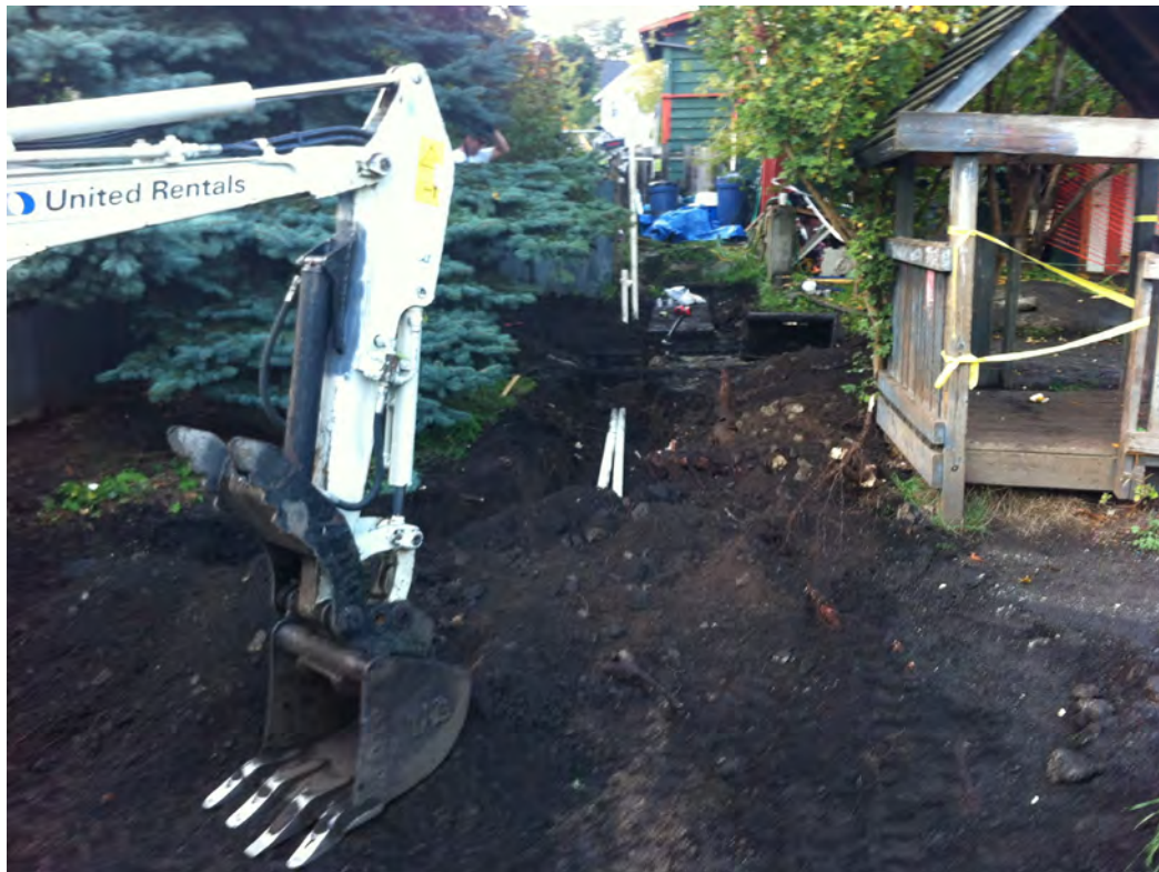
Figure 4.29: The underground pipes leading into the play area
