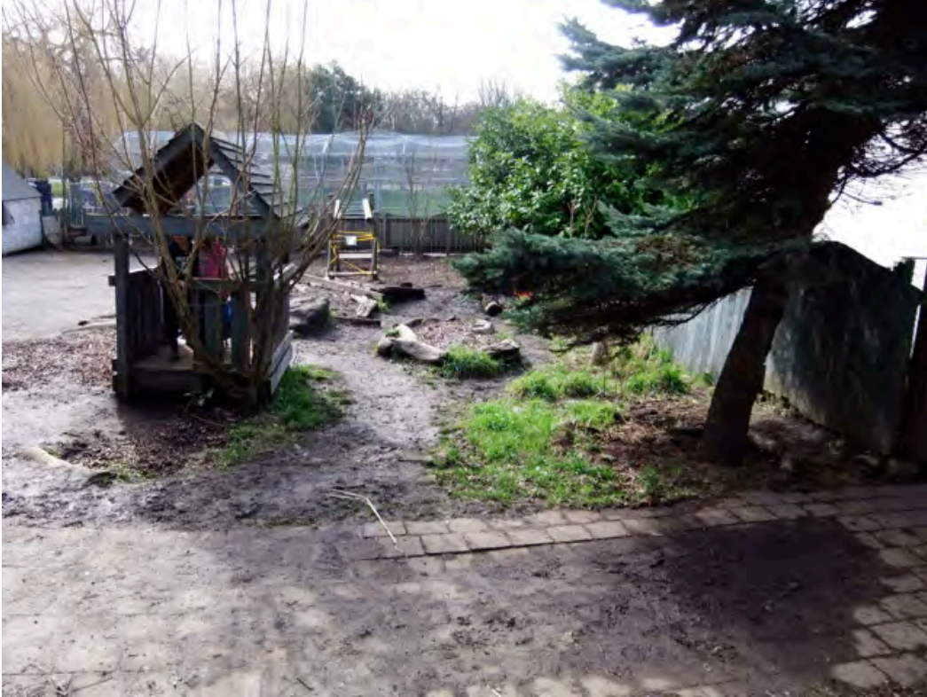
Figure 4.8: Site photo 4: Looking south at the play area with poorly graded pathway in front
