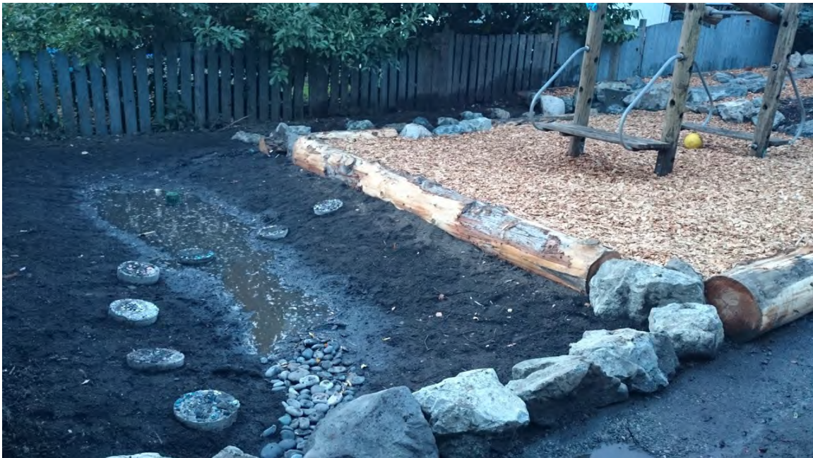
Figure 4.37: The completed stepping stones placed in the rain garden before it was planted
