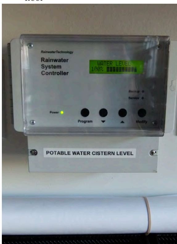
③ Figure 3.8: Water monitor system for the “potable” rainwater tank
