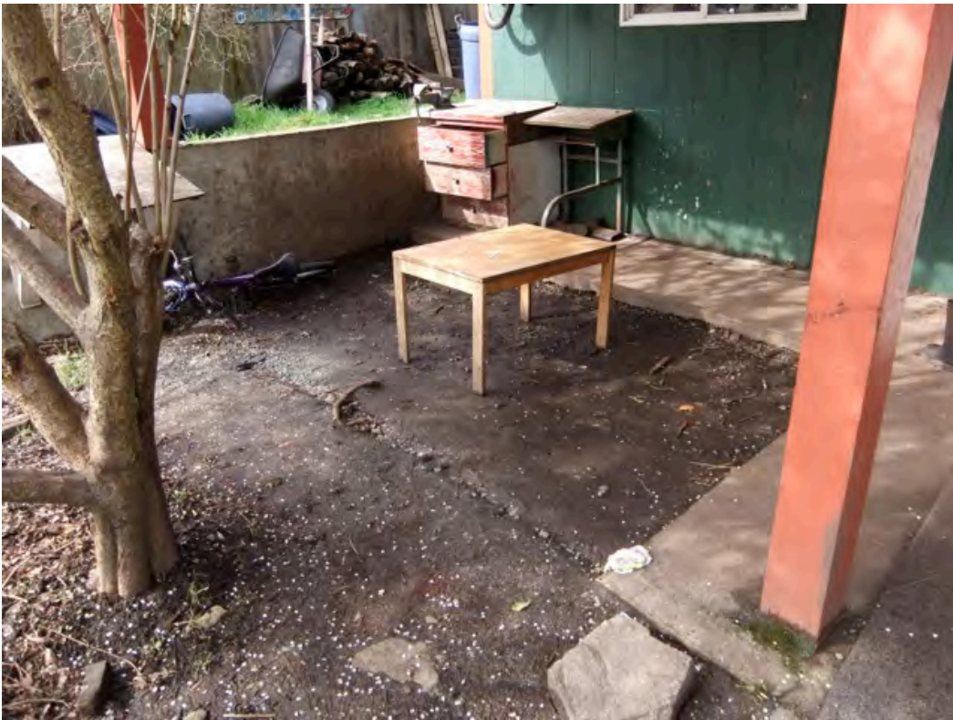
Figure 4.9: Site photo 5: Covered seating area below deck with visible water drip line
