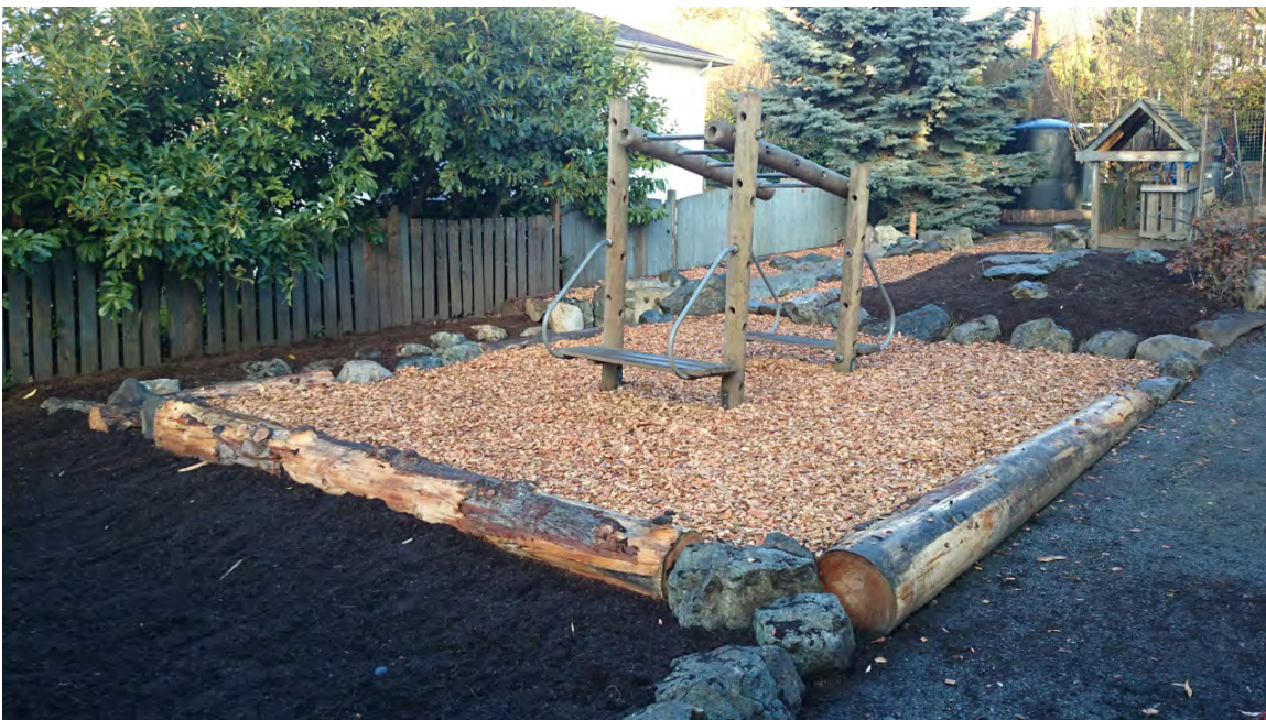
Figure 4.52: The entire play area and gardens were rebuilt and the monkey bars were reinstalled.
