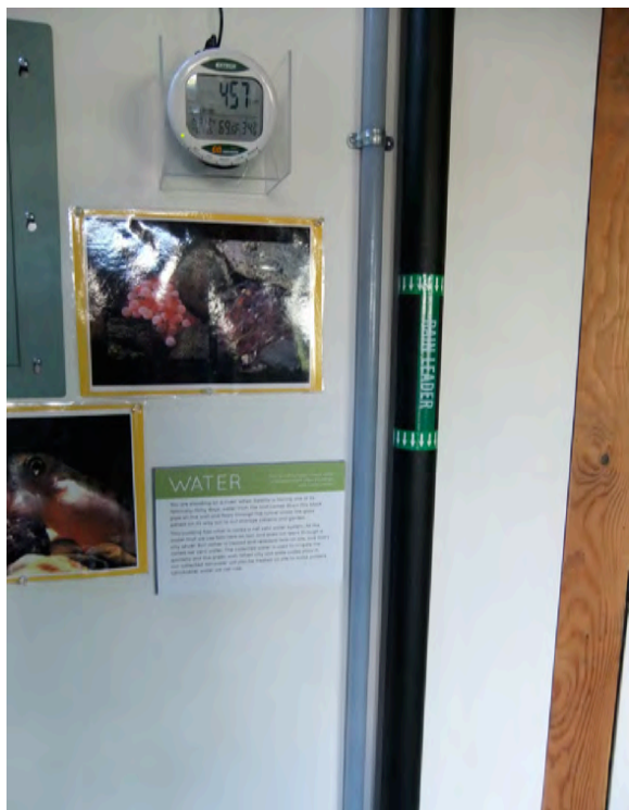
① Figure 3.6: Rainwater leader coming from the roof into the runnel in the floor
