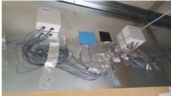
Figure 11. Typical data logger and sensor installation
