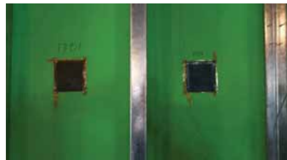
Figure 3. Interior Heat Flux Sensor Installation
