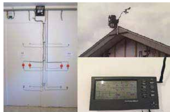
Figure 3: Interior sensor installation and weather station.
