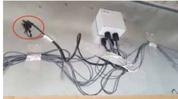
Figure 13. Differential pressure sensor installation
