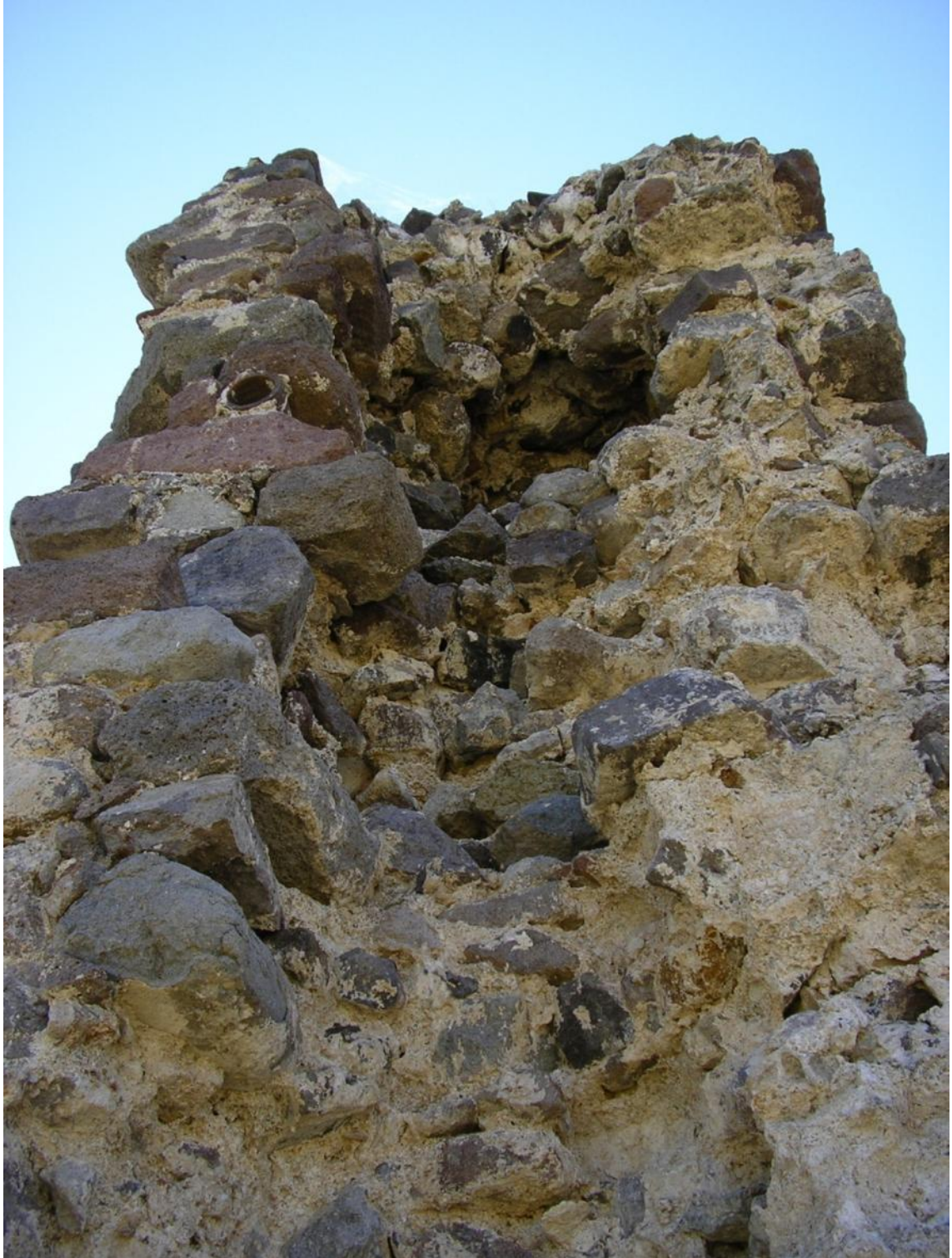
Figure 7.4: View of Vertical Groove on WNW-Side of Tower
