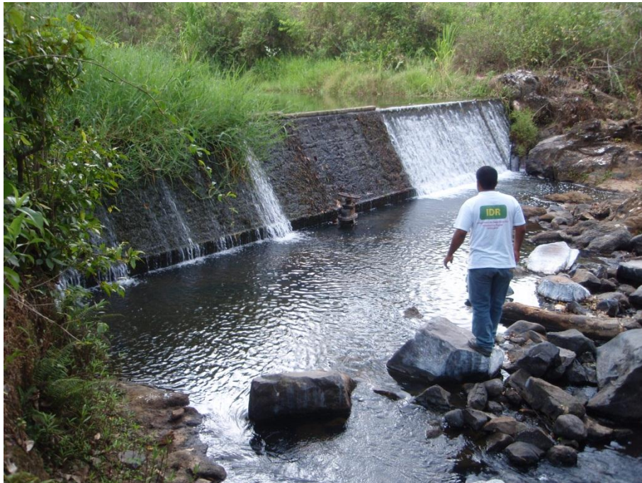
Figure 3-1. Drinking water intake for La Libertad
