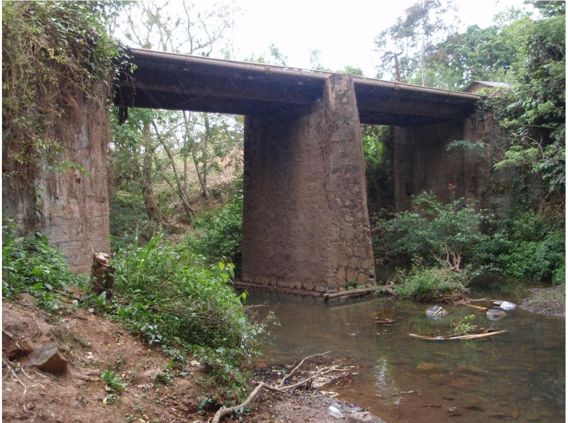
Figure 4-3. La Libertad bridge. Sample site SW-17/I-05 is on far (downstream) side of bridge.
