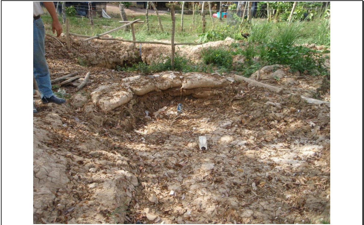
Figure 2-5. Settling pond downstream of a rastra in La Libertad. The pond was dry as the photograph was taken during the dry season.
