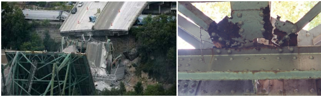
Figure 1.6: Collapse of the I35W Mississippi River bridge [6].
