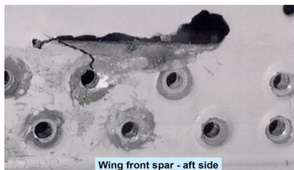
Figure 1.4: Fatigue crack developed by corrosion in wing front spar joint.
