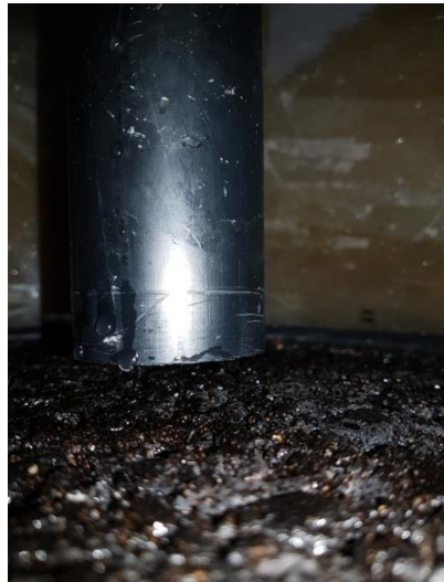
Figure 6 Gap of 0.5 inch between pavement and open end of the pipe
