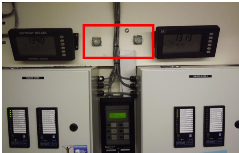
Figure 5: Diagnostics Ports in Underdeck Control Room
