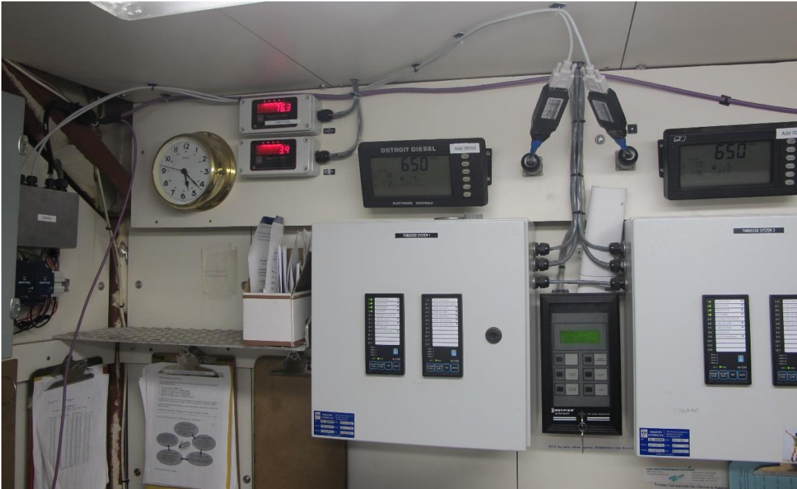
Figure A-1: J1587/1708 Engine Bus Connection in Control Room
