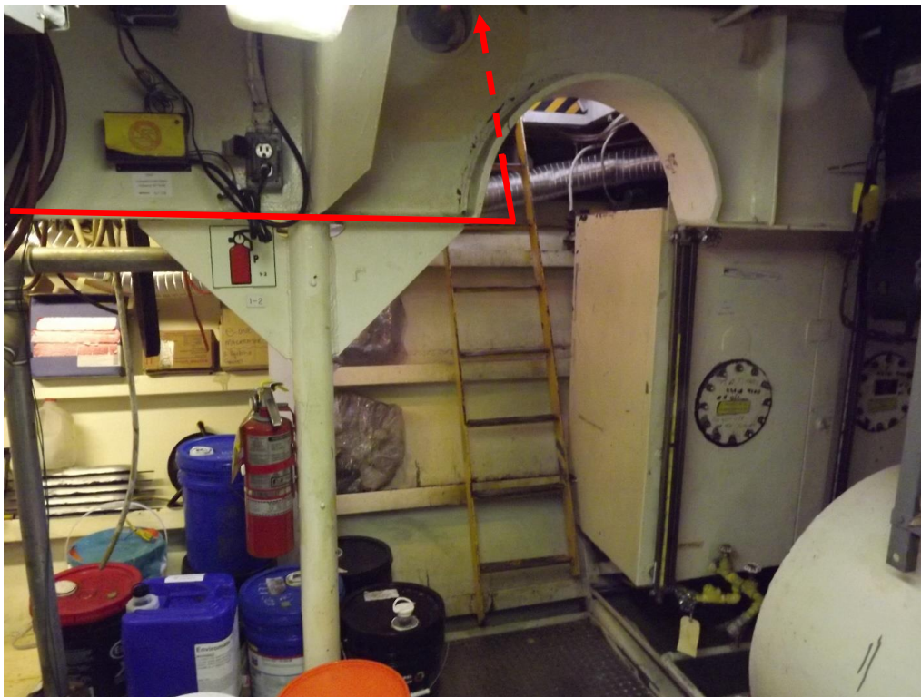
Figure 22: Cable Routing Up Stairwell from Lower Deck Heading Towards Cabin Rooftop
