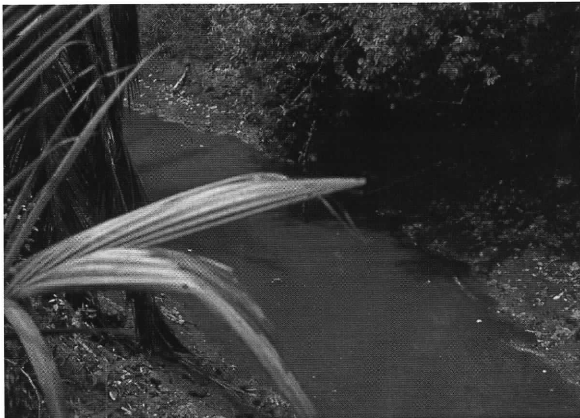
Figure 6.8 Small Irrigation Canal Occluded by Shrimp Farm Sediment
