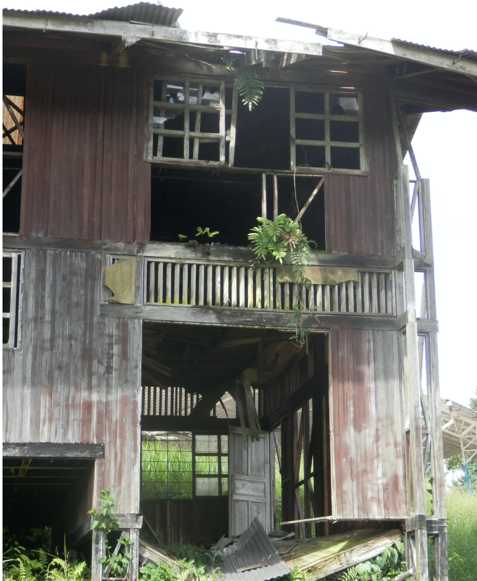
Figure 7.22. Damaged building at CONFENIAE's headquarters in Unión Base, photo by Nicolás.
