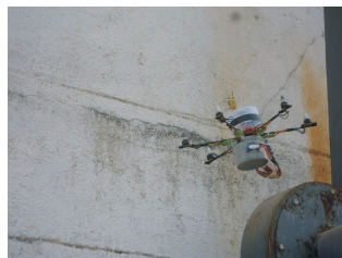
(b) Closer Examination of Cracks
