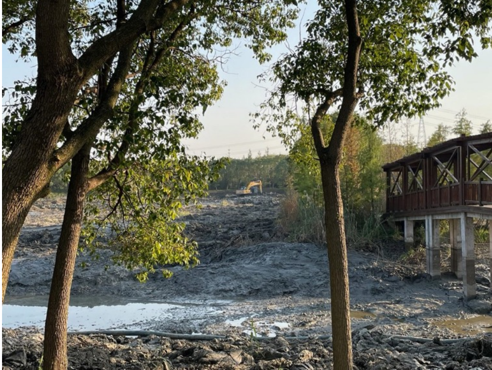
Figure 1.2 A digging machine working in the middle of the wetland construction site in Tongli National Wetland Park (photo taken by the author).
