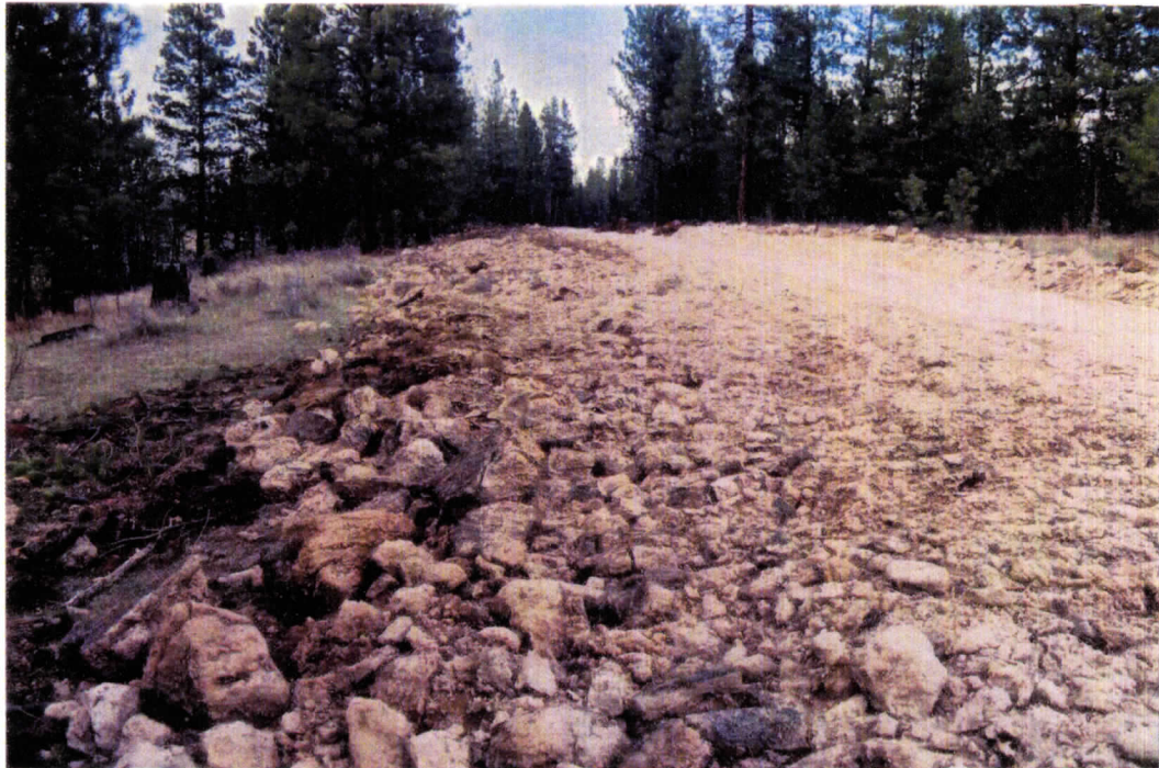
Figure 78: Large expanse of overburden on west side of upgraded FSR, looking north
