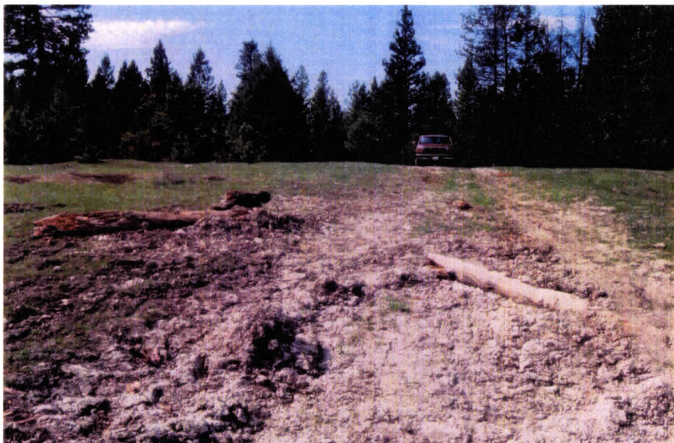
Figure 88: Condition of road surface following disturbance, looking south to knoll
