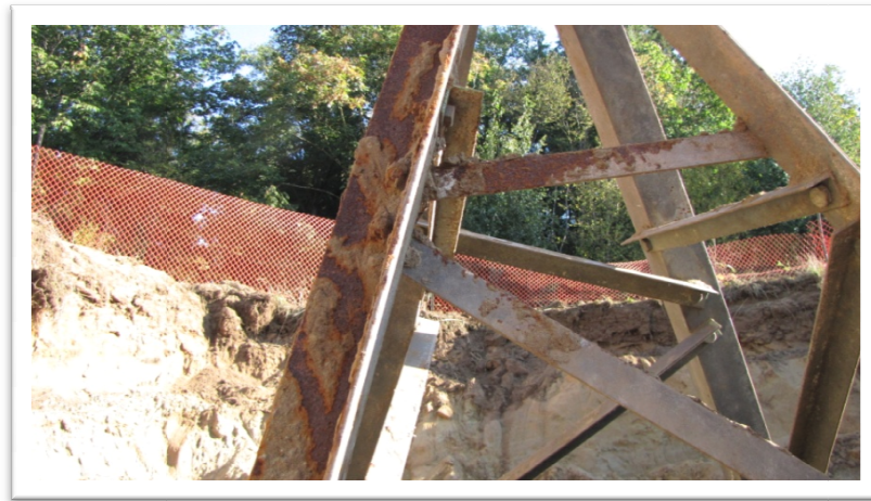
Figure 46 – Corroded tower leg at location B
