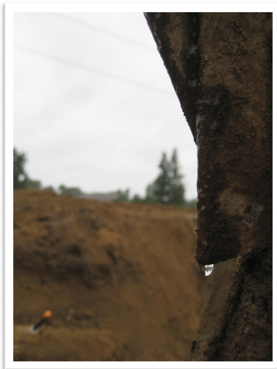
Figure 45 – Moisture accumulation during rain storm on transmission tower at location D
