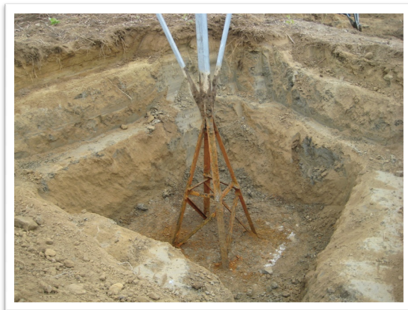
Figure 47 – Corroded tower leg at location D. Notice the contrast between above ground and subsurface steel corrosion.
