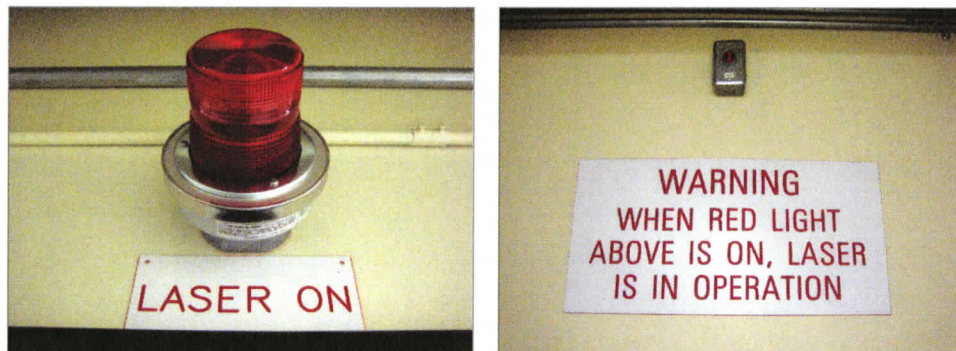
Figure 2.2.3: These impressive-looking light fixtures let the user know that the laser is in operation. Not only do they warn users of radiation danger, but they also provide feedback to the user, showing that the laser has been engaged.
