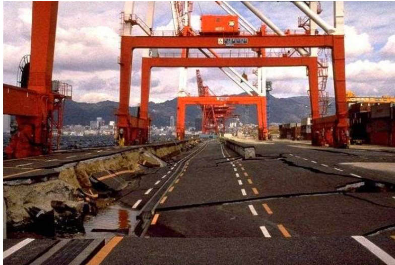
Figure 1-3 Lateral displacement of a quay wall on Port Island, Kobe 1995. (Werner et al. 2011)
