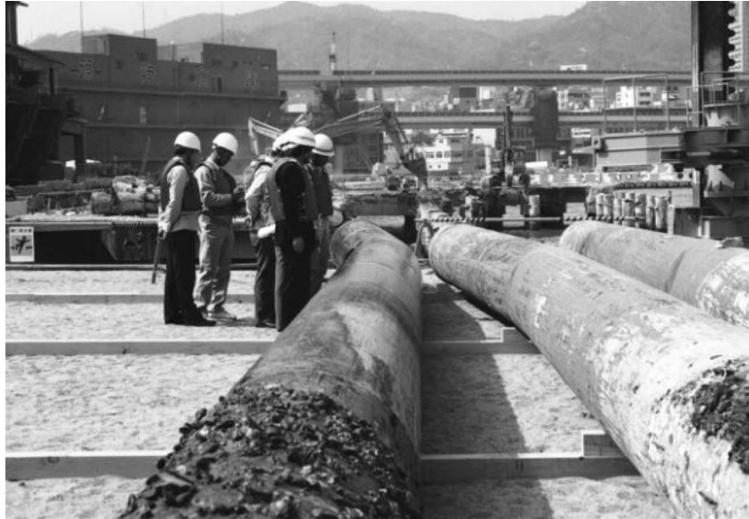
Figure 1-5 Damage to piles at Takahama Wharf, Kobe Port (after extraction for inspection). (PIANC 2001)
