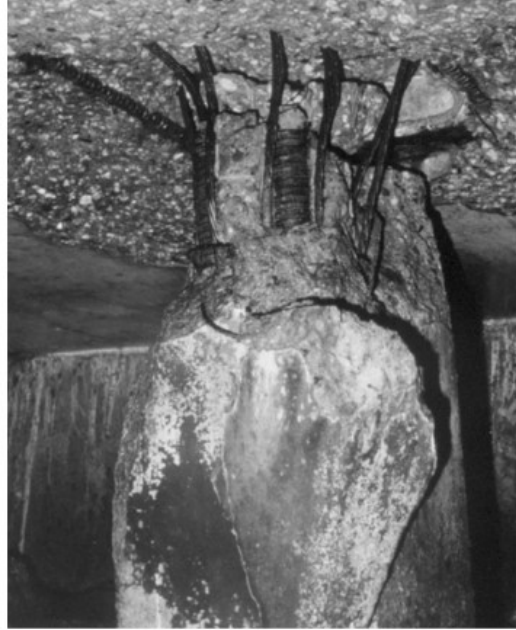
Figure 1-2 Damage at a pile-deck connection, Loma Prieta earthquake 1989; Ben Nutter Terminal Wharf, Berths 35 – 37. (Serventi et al. 2004)
