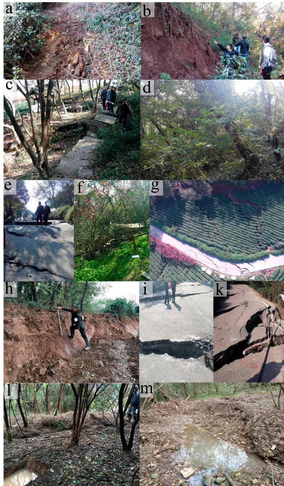
Figure 4. (a) Scarp on the trailing edge of landslide, photographed 23 September 2016; (b) scarp on the trailing edge of landslide, photographed 3 November 2016; (c) broken mountain road; (d) toppled trees; (e) cracks on Dlinglin Road; (f) deformation of retaining wall; (g) groove on the northwest side of landslide; (h) subsidence of groove [16]; (i) cracks on Zulong Road; (k) cracks on Dinglin Road; (l) front shear outlet; (m) groundwater flowing out of the surface, their positions are shown in Figure 5.
