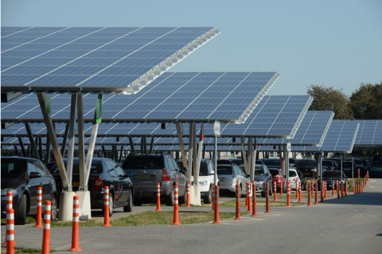
Figure B3. A solar carport installation at the Weeze Airport in North Rhine-Westphalia, Germany (Ola, 2016, Figure 2).
