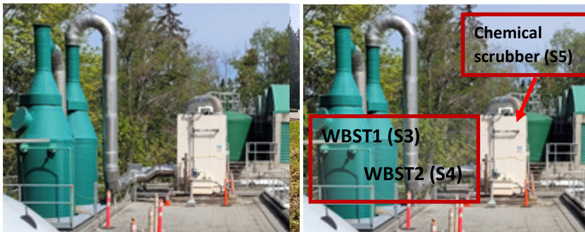
Figure 15: (Left) Photo of the covered ATADs, (Middle) ATAD foul air sample location S1, (Right) Photo of WBSTs and Chemical scrubber at WWTP1.
