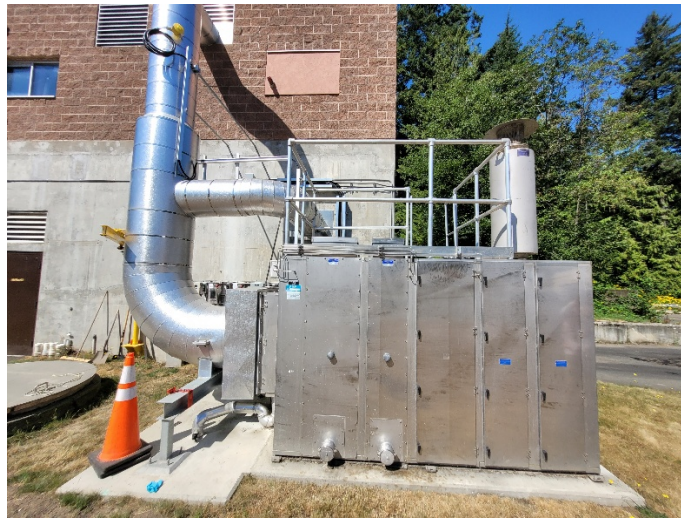
Figure 19: Photo of modular carbon scrubber used to treat foul air for biosolid de-watering process at WWTP2.
