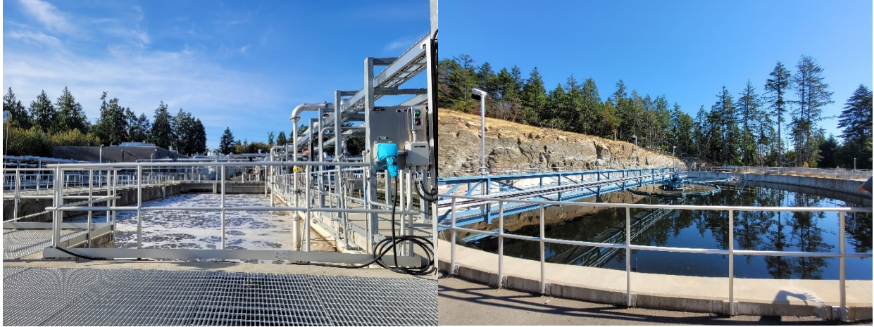
Figure 22: (Left) Photo of secondary water treatment system aeration tanks. (Right) Photo of clarifiers at last step before water discharge to environment.
