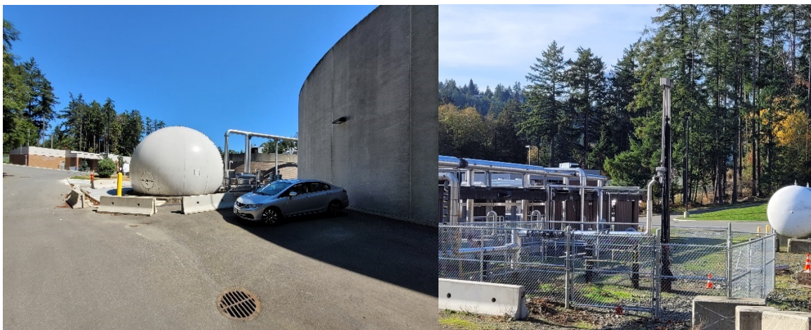
Figure 20: (Left) Photo of biogas storage ball. (Right) Photo of flare onsite WWTP2.
