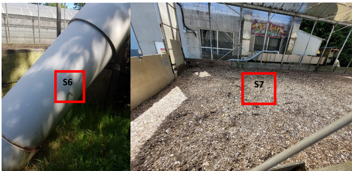
Figure 16: (Left) Photo of ductwork exhausting the de-watering room and sample point S6. (Right) Photo of biofilter and sample location S7 at WWTP1.
