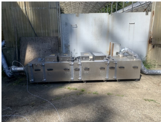
Figure 17: Photo of temporary demonstration advanced oxidation unit for odour control to treat exhaust air from de-watering process at WWTP1. Air was sampled at the inlet on the left of unit and outlet at the right (May/June 2022).
